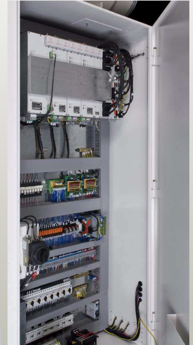
Electric System For Easy Maintenance
