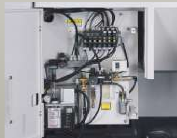
Hydraulic & Lubrication System(LU-620)
